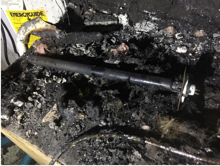
Exhibit A Charred Unit
