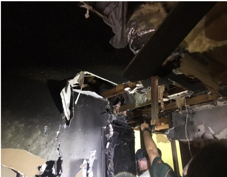
Exhibit B House Damage
