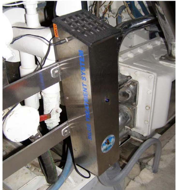
Holding Tank Ventilation System
